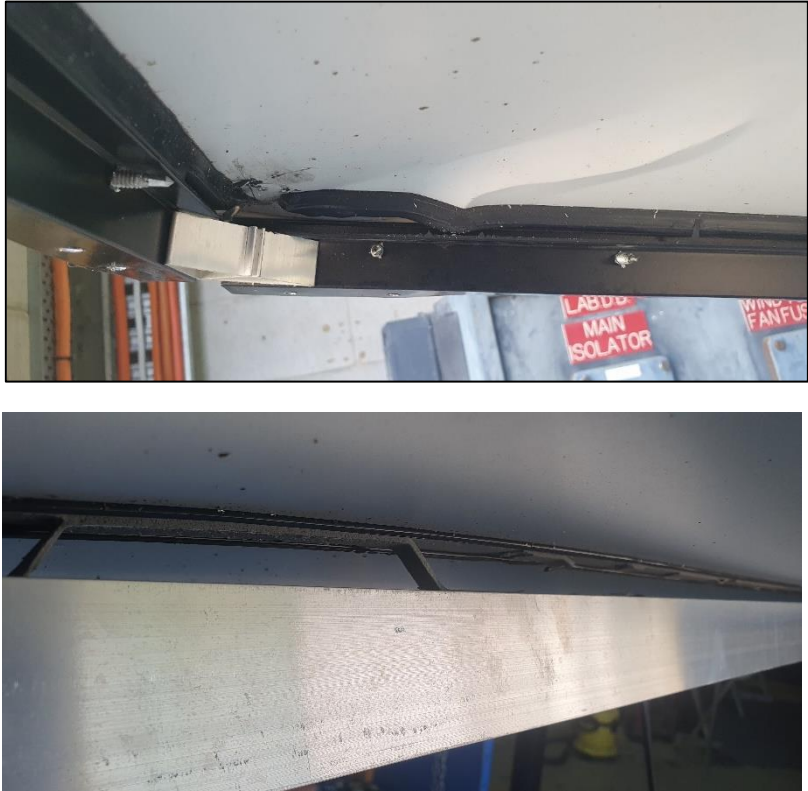
Figure 9: Typical deformation of skin viewed from underside of panel (upper) and view of detachment of stiffeners from underside of panel (lower)
